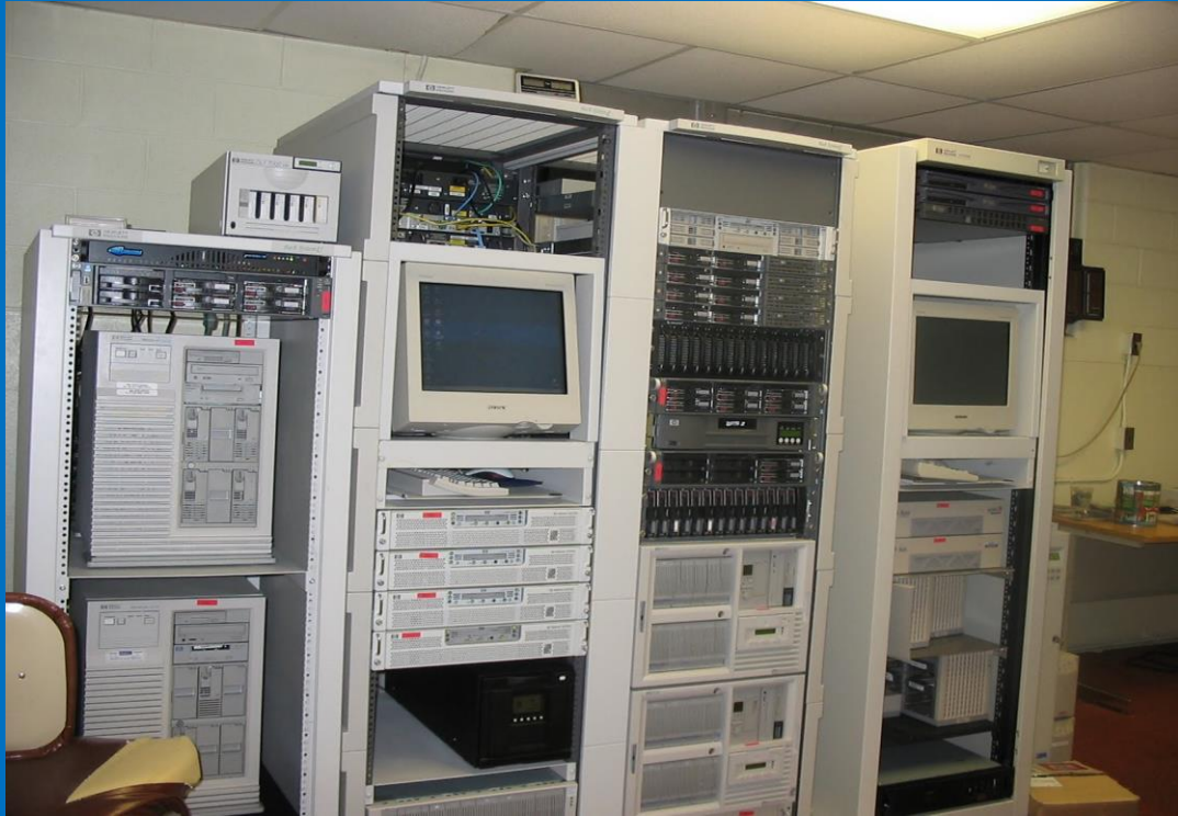
Servers Room On premise Datacenter
